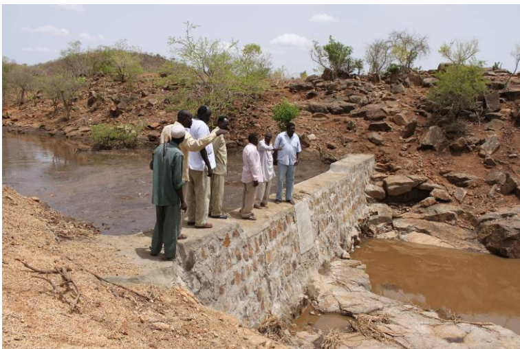
Sand Dam constructed by local apprentices (trained by SOS Sahel) on the Marui River, Damba Village, South Kordofan, June 2010.
